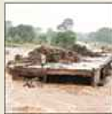
A washed away bridge in Chimanimani, Zimbabwe. Reuters
