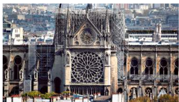
A damaged section of the Notre-Dame Cathedral. •REUTERS
