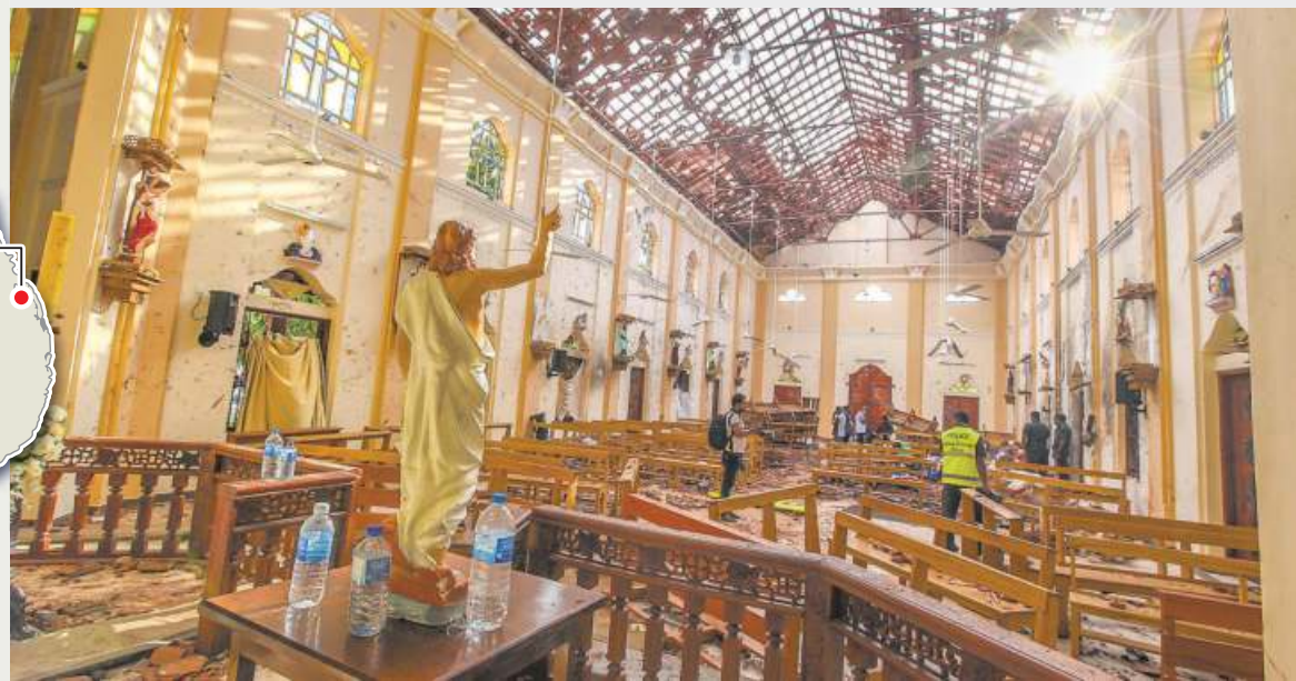
Broken calm: A view of the St. Sebastian's Church in Negombo, north of Colombo, which was damaged in a blast on Sunday. ■ AP
