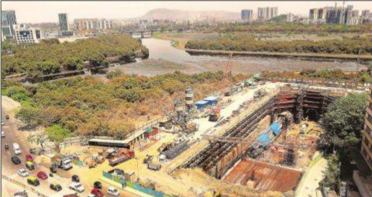
Metro construction in progress near the Mithi, as seen from BKC. Pradip Das
