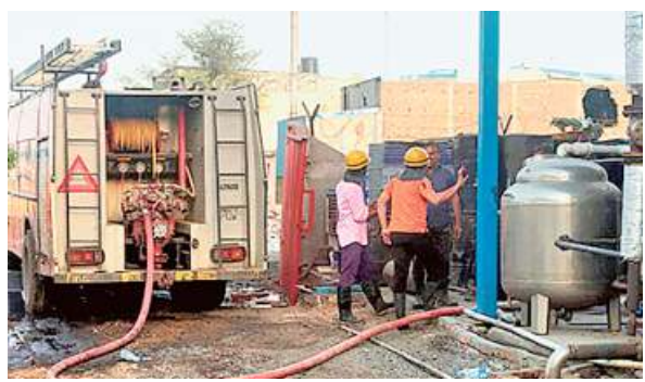
Fire department personnel at the Nuh plant. ■ SPECIAL ARRANGEMENT
