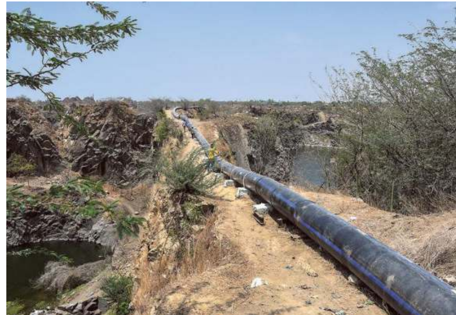
Vital link The giant pipes drawing water from quarries in Sikkarayapuram to the Chembarambakkam treatment plant.
