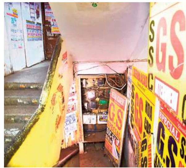
(Far left) Electric cables hanging precariously at one of the coaching centres; and a view of the coaching institutes in Mukherjee Nagar. ■ SUSHIL KUMAR VERMA
