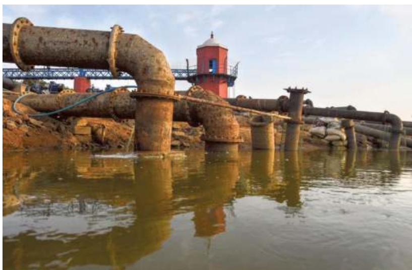
Plumbing the depths With storage at Red Hills reservoir dipping to its lowest level, Metrowater is pumping dead storage through giant pipelines to supply the city.
