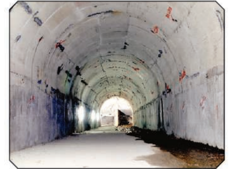
THE TUNNELS OF THE PROJECT ARE WIDE ENOUGH TO HAVE TWO CARS DRIVE BY SIDE BY SIDE
