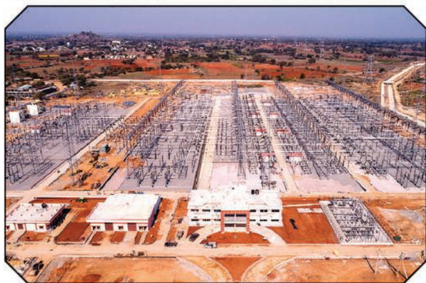
THE PACKAGE - 11 SUBSTATION
