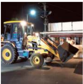
Earthmovers being pressed into service to pull down Praja Vedika at Undavalli.
