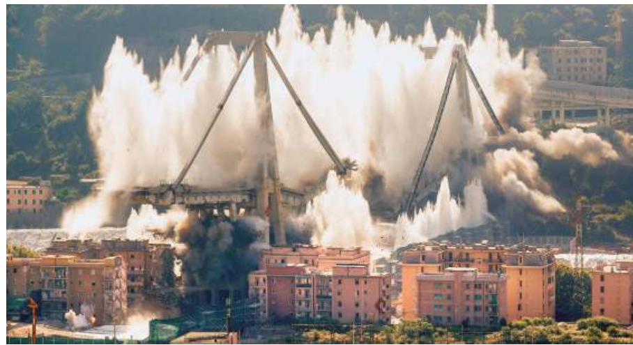
Done and dusted: A cloud of dust rises as the remaining spans of the Morandi bridge, which collapsed nearly a year ago killing 43 people, were demolished in Genoa, Italy, on Friday. AP
