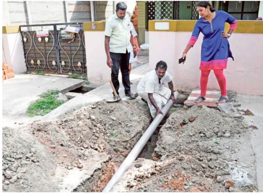
For connecting several such houses to the underground sewerage scheme, the Coimbatore Corporation has borne the beneficiaries' cost. - M. PERIASAMY
