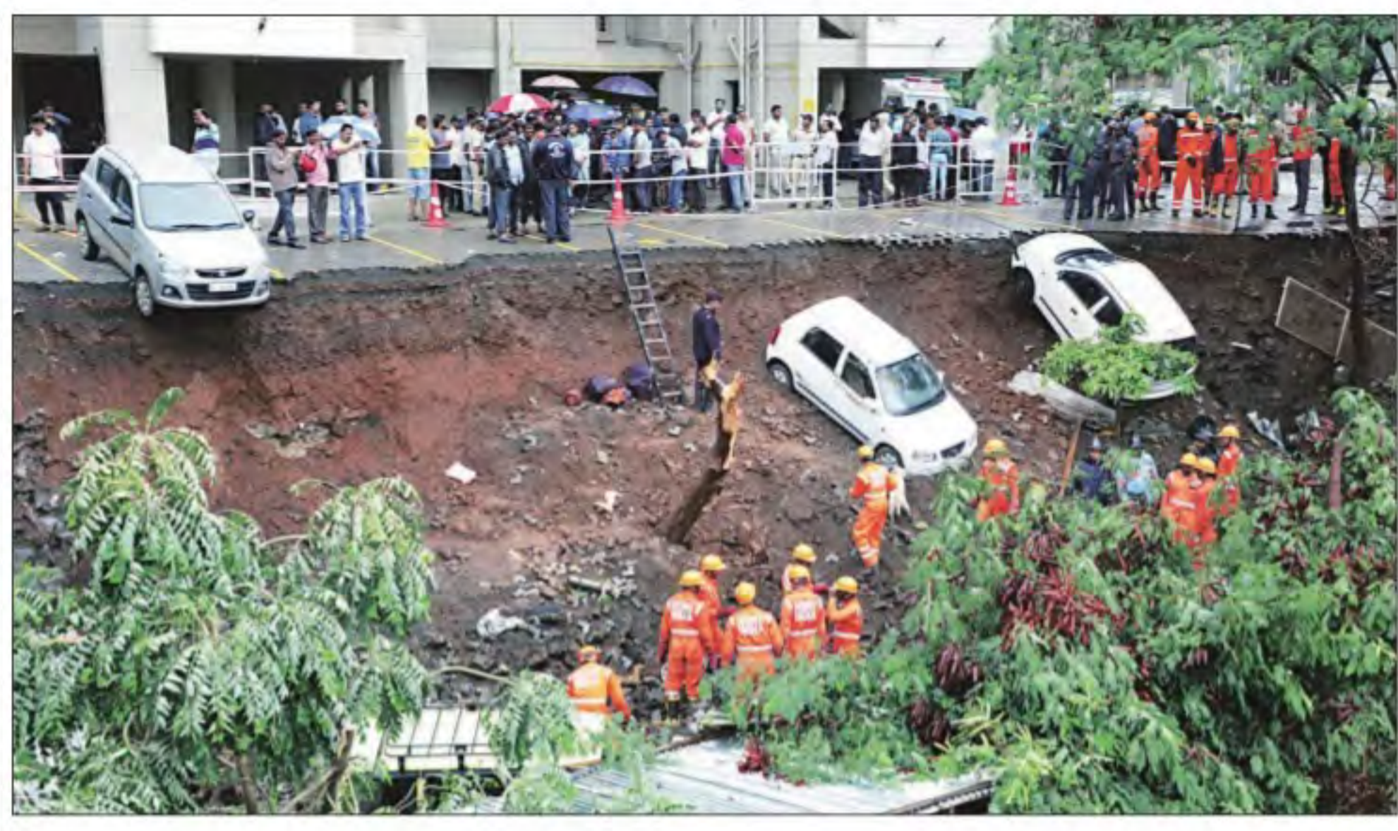
The site of the wall collapse in Pune on Saturday. The victims were construction labourers and their relatives. Arul Horizon
