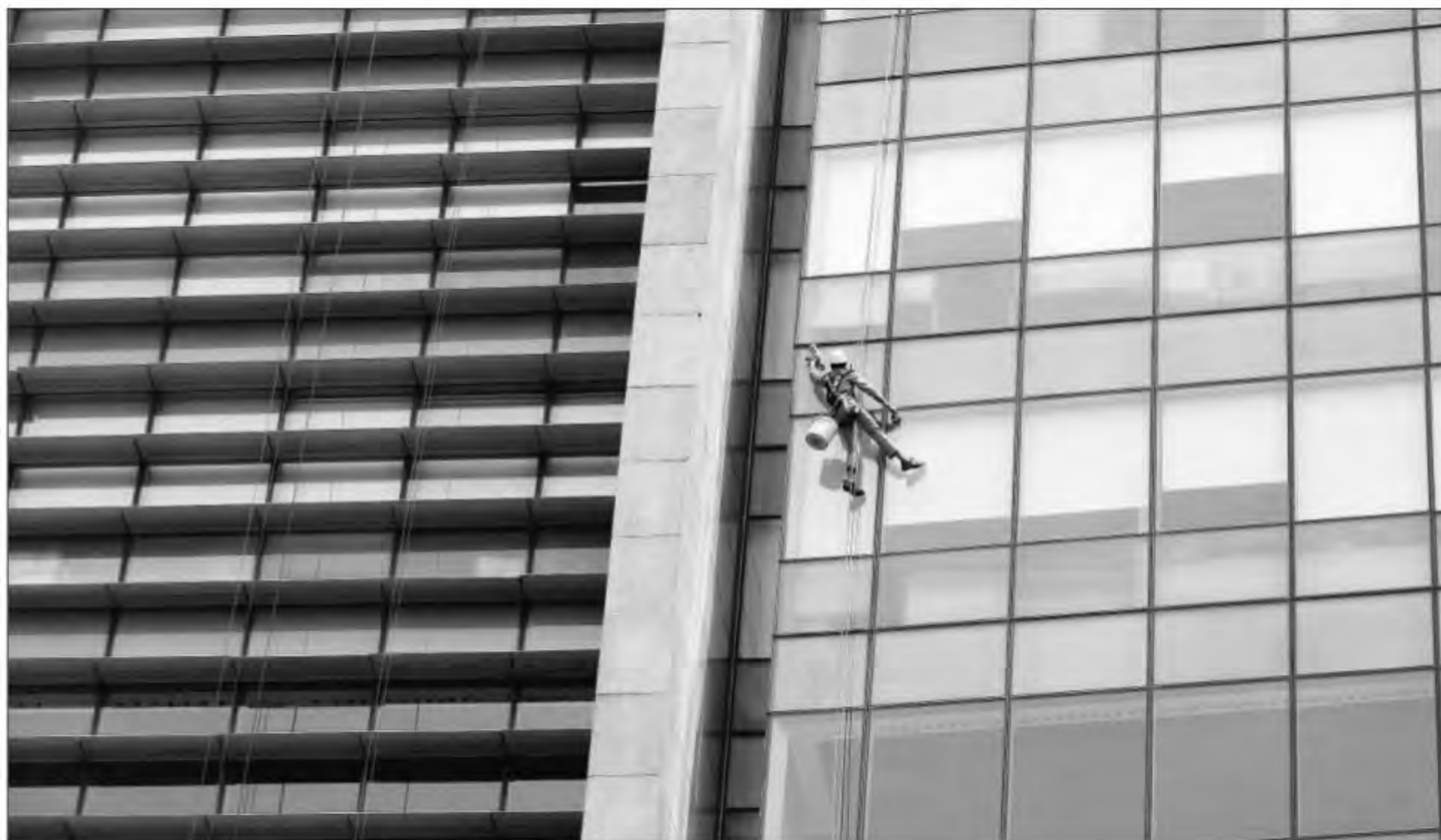
Shailendra Yadav cleaning the glass facade of the 14-storey Vatika City Point in Gurgaon. One round, all the way down, takes about 45 minutes. Photos by Gajendra Yadav
