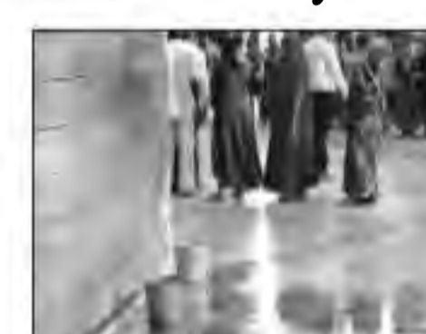
Buckets kept at the exhibition hall after roof started leaking. Bhupendra Rana
