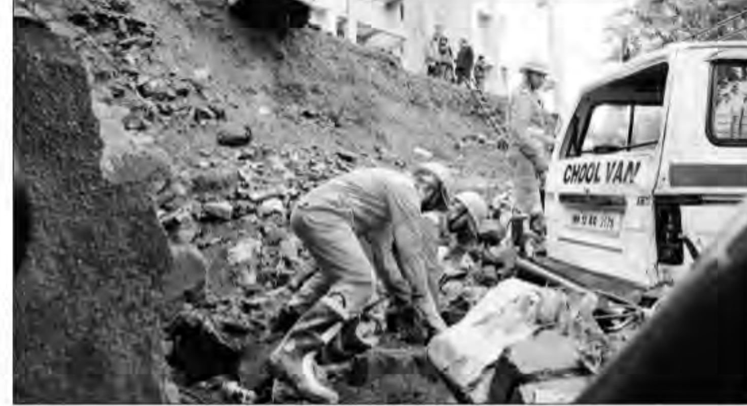
Rescue personnel at the site of the wall collapse in Pune on Saturday. Arul Horizon
