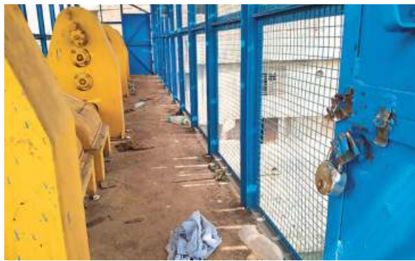
The broken lock of the room which has the controls to the gates. *SPECIAL ARRANGEMENT
