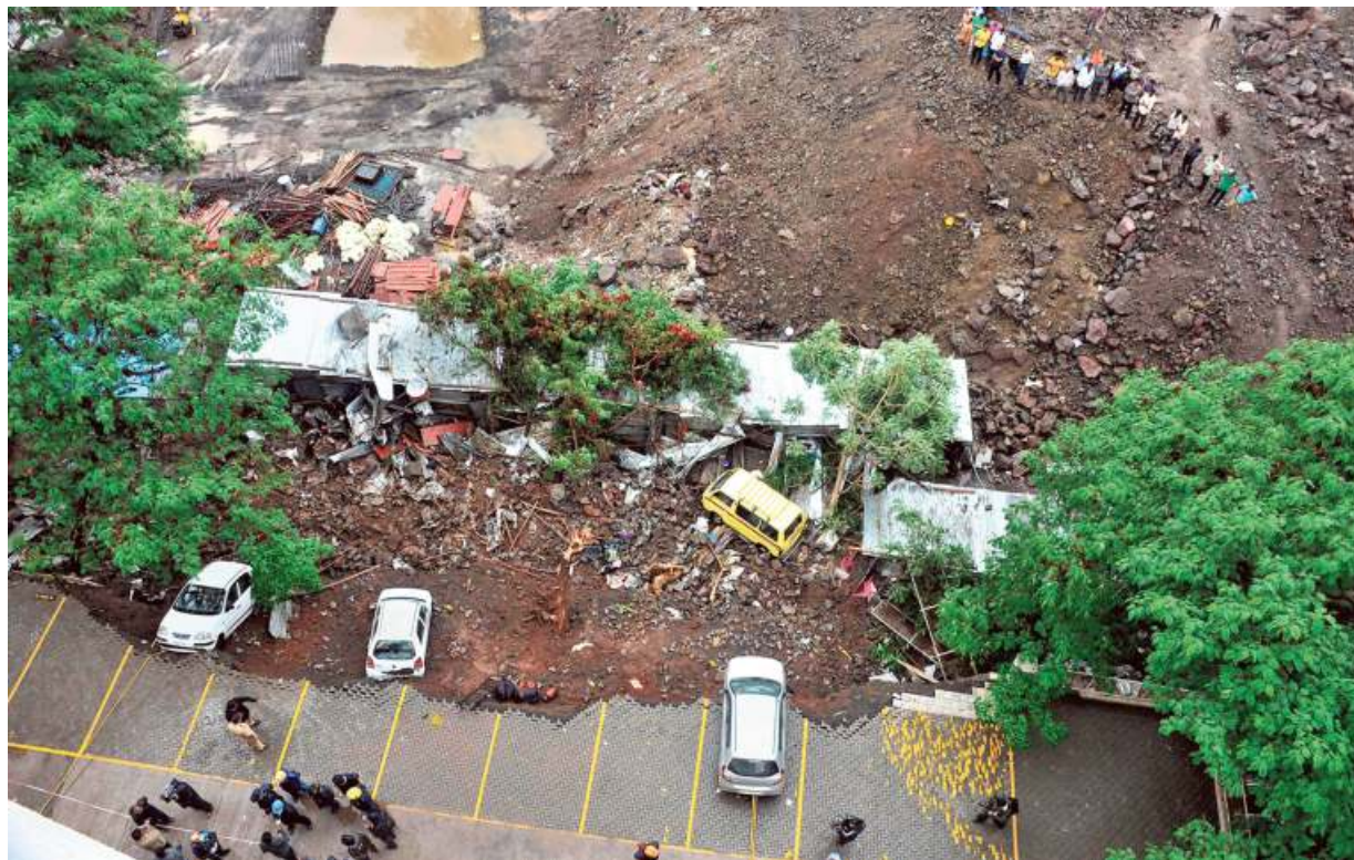
Buried under: As rain pounded Pune, 15 persons, including four children, were killed when a part of a compound wall of an apartment complex crashed on workers' hutments at Kondhwa on Saturday. The deceased hailed from Bihar. *PTI (PAGE 9)
