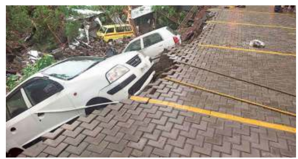
Caved in: Dislodged cars at the site where the compound wall of a housing society collapsed on Saturday. •PTI
