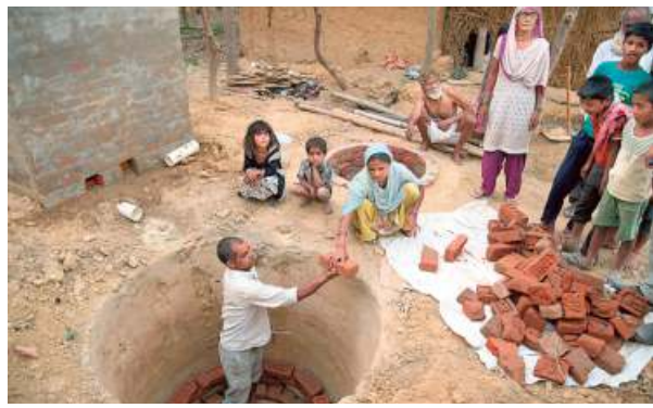
Brick by brick: A file photo of a man building a toilet under the Swachh Bharat Abhiyan in Gonda, Uttar Pradesh. ■ RAJEEV BHATT
