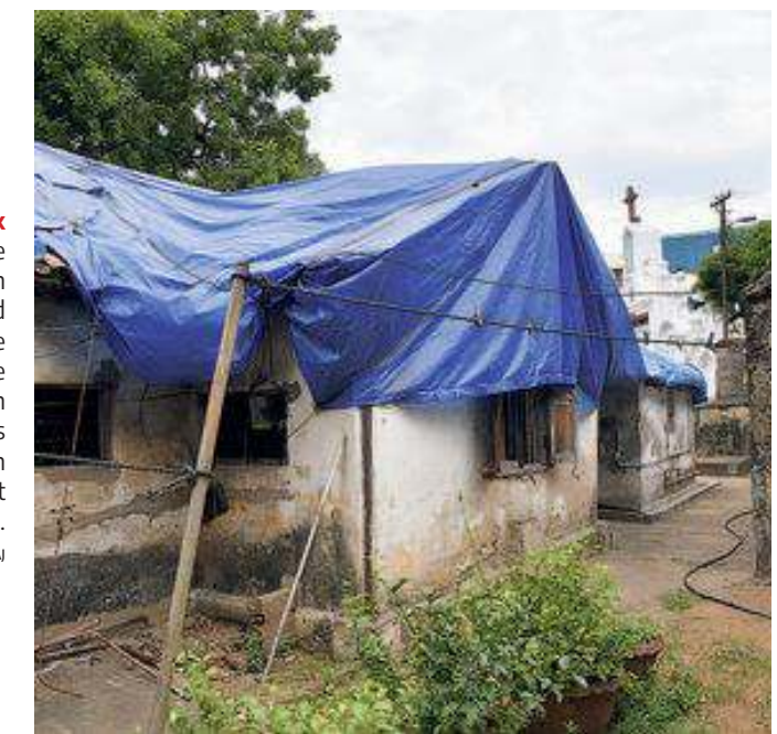
Tough task Maintaining heritage homes is an extremely cash- and labour-intensive affair. This once church-owned house in St. Thomas Mount is covered in tarpaulin to protect it from rain. B. VELANKANNI RAI
