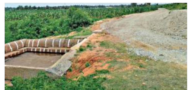
The World Heritage Committee was concerned about a proposal to widen the road near the tank area in Hampi.
