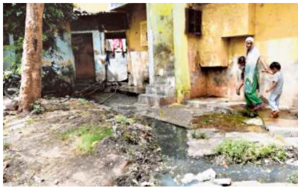
Water woes: Sewage spilling out of dug-out drains at the Jeevan Jyoti colony in Bhopal on Saturday. ■ A.M. FARUQUI
