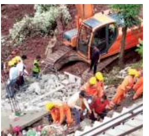
NDRF men undertake rescue work at the site of a building collapse in Solan. *PTI
