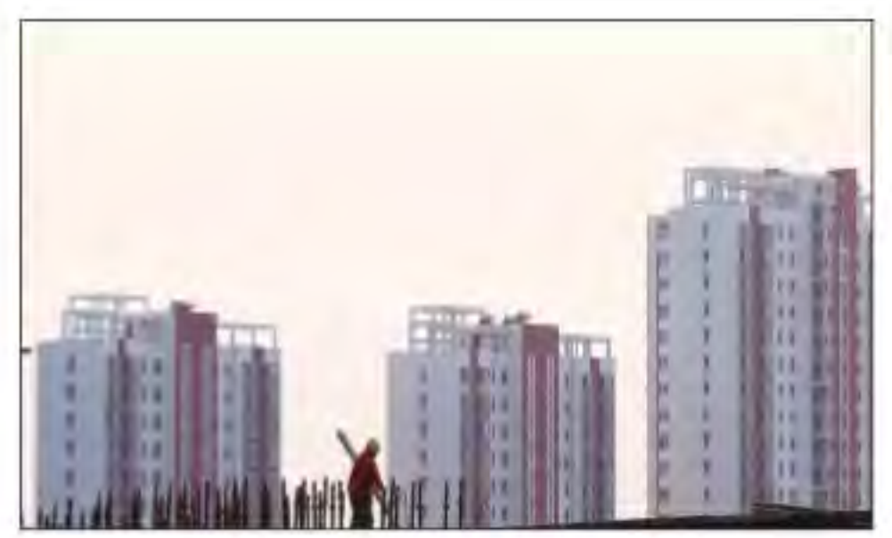
A construction site in Huaian. Growth in China's new home prices cooled in June as sales shrank for a 2nd month. Average home prices in 70 cities grew 0.6% in June from a month earlier, easing from a 0.7% in May, according to Reuters calculations based on National Bureau of Statistics data. Reuters file photo
