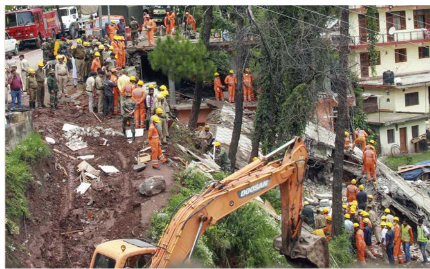
Rescue and relief work underway after a building located on the Nahan-Kumarhatti road which housed a restaurant collapsed on Sunday evening after heavy rain in Solan district, Himachal Pradesh, on Monday. — PTI
