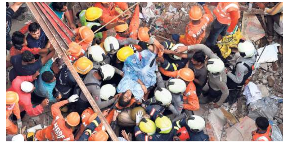
Lucky escape: Rescue personnel with a woman who was pulled out of the rubble after a four-storey building collapsed in the Dongri area of Mumbai on Tuesday. Ten persons were killed and over 40 are feared trapped. ■ VIVEK BENDRE (REPORT ON PAGE 9)
