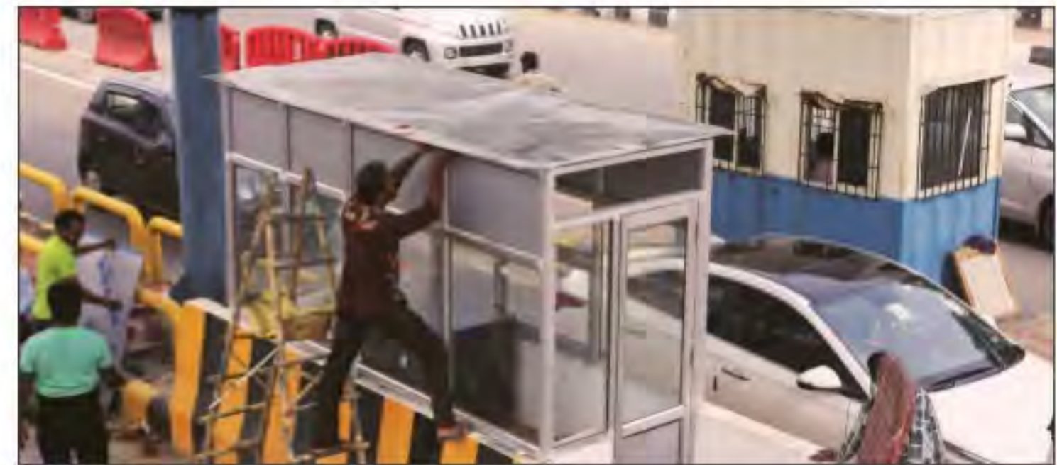
RFID tag cabins being constructed at Ghazipur (main) toll plaza, Tuesday. Abhinav Saha
