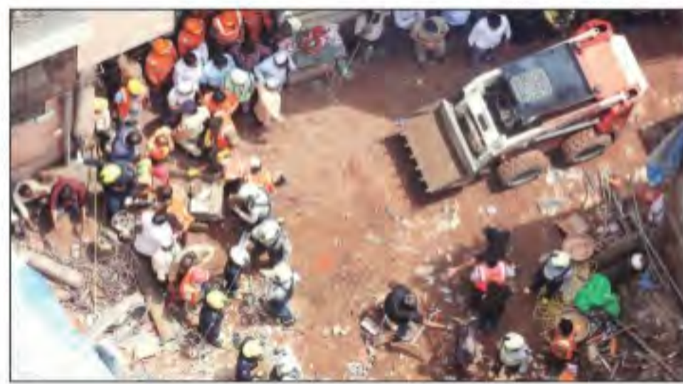
Rescue work in progress at the site of the building collapse in Dongri, on Wednesday. Prashant Nadkar
