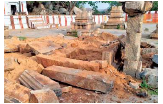
Erasing history: The vandalised 'Brindavan' of Sri Vyasaraja Tirtha on the Tungabhadra banks. *SPECIAL ARRANGEMENT
