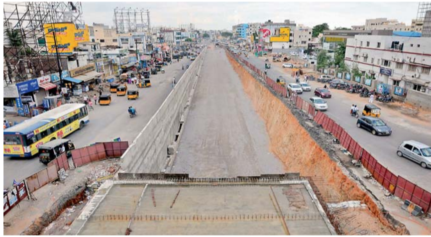
The work of the under-construction Road Under Bridge connecting Nagarjunasagar Ring Road with Secunderabad which is at a brisk pace is expected to provide a big relief to the motorists. — P. SURENDRA
