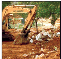
Illegal drilling of rocks at Fakharudindutta on Saturday
