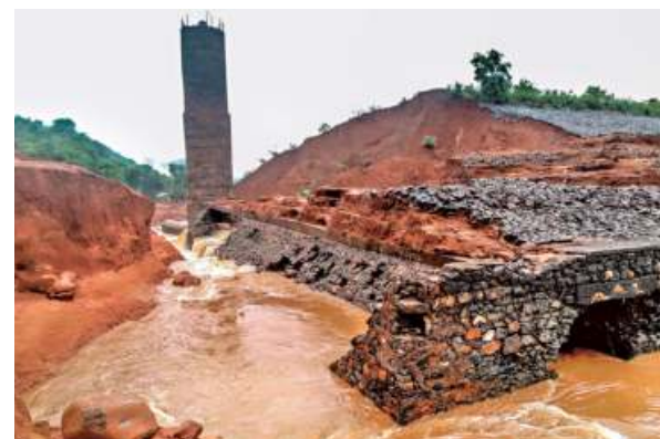
Force of nature: Water flowing out of the breached Tiware dam in Ratnagiri district of Maharashtra. • RAJU SHINDE
