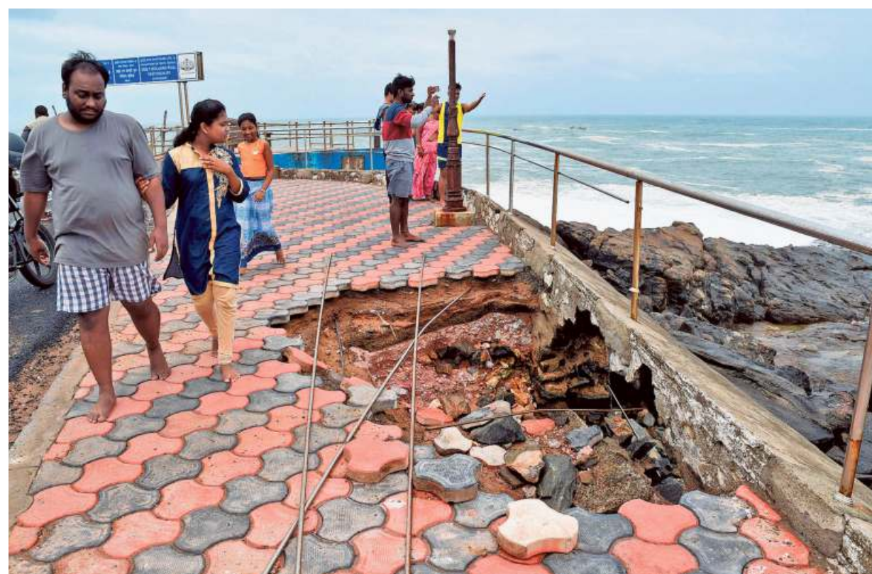
Obstacle course: Sea erosion has left a gaping hole in a walkway in the coastal town of Vizhinjam in Kerala. The walkway is close to the Bollard Pull Test Facility, which is used to check the tugging capacity of ships. ■ S.GOPAKUMAR
