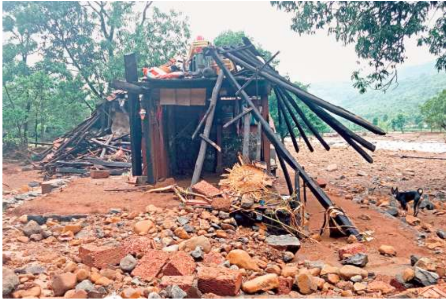
Trail of misery: A house at Tiware village, which was damaged following a breach in Tiware Dam in Ratnagiri district on Tuesday night after heavy rain. • RAJU SHINDE
