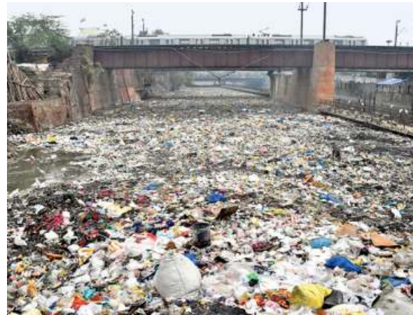
Sordid state: Garbage clogging a drain near the Seelampur area in New Delhi. ■ R.V.MOORTHY
