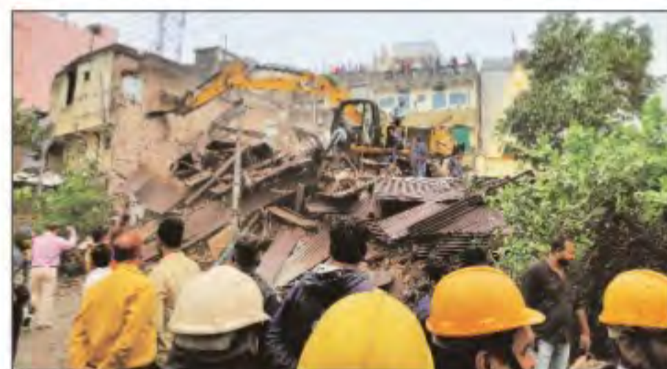
The building was declared a safety hazard. Dipankar Ghose
