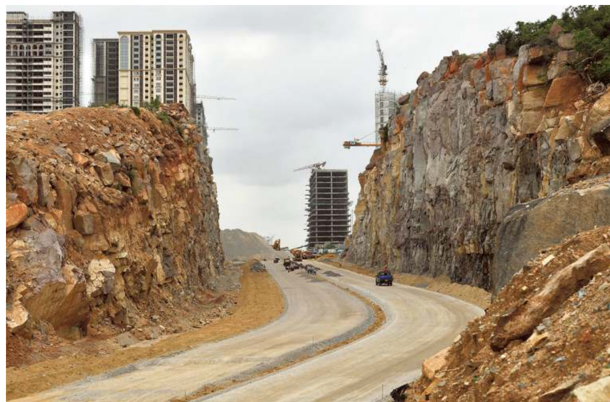
Paving the way: A road has been laid by breaking a hillock beside the Biodiversity Park at Gachibowli in Hyderabad. The road leads to the towers built on the other side. ■ G. RAMAKRISHNA
