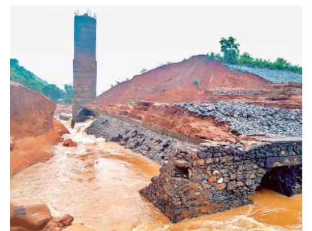
A view of the Tiware dam which breached last week following incessant rains in Ratnagiri, causing a flood-like situation in seven downstream villages. •FILE PHOTO
