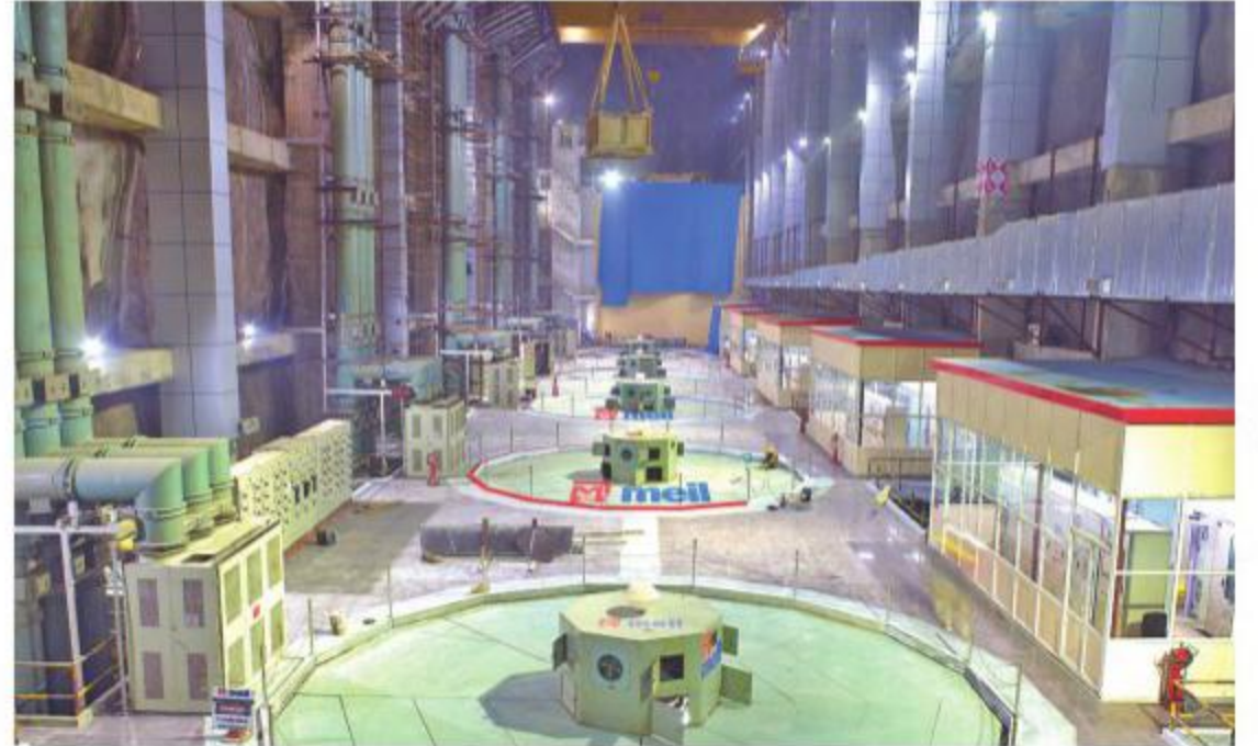
Officials successfully conducted the wet run of the fifth machine at Laxmipur underground pump house of Kaleshwaram Lift Irrigation Scheme for the second day on Monday | EXPRESS
