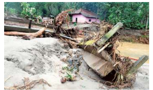
Rain fury: A damaged bridge at Kakkineji in Dakshina Kannada district of Karnataka. *H.S. MANJUNATH
