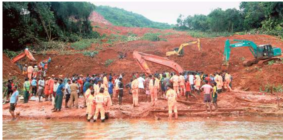
Tough task: Work being carried out at the landslide site in Malappuram. *SAKEER HUSSAIN
