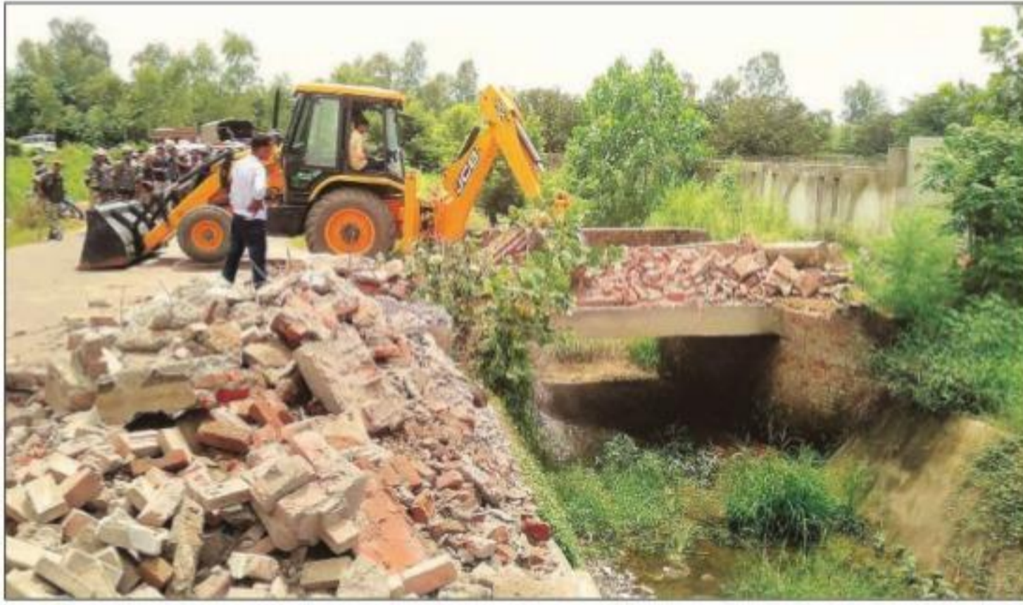
Rampur district administration officials demolish the boundary wall of the resort in Rampur on Friday. PTI
