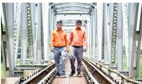
Special sense: Two gangmen checking the tracks on a railway bridge. •SPECIAL ARRANGEMENT
