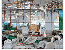
A damaged stage of a wedding hall after a blast in Kabul on Sunday
