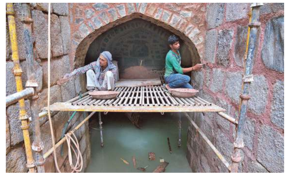
Construction work in progress at the baoli within Humayun's Tomb. ■R.V. MOORTHY
