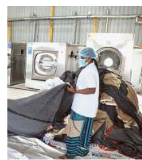
A file picture of Railway laundry facility in Tirupati. K.V. POORNACHANDRA KUMAR
