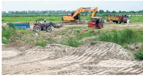
The shallow reservoir was supposed to be completed by August 20. • FILE PHOTO: SANDEEP SAXENA
