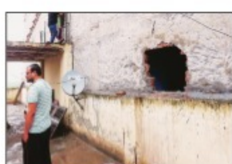
The wall on the terrace of the adjacent house was broken to rescue people
