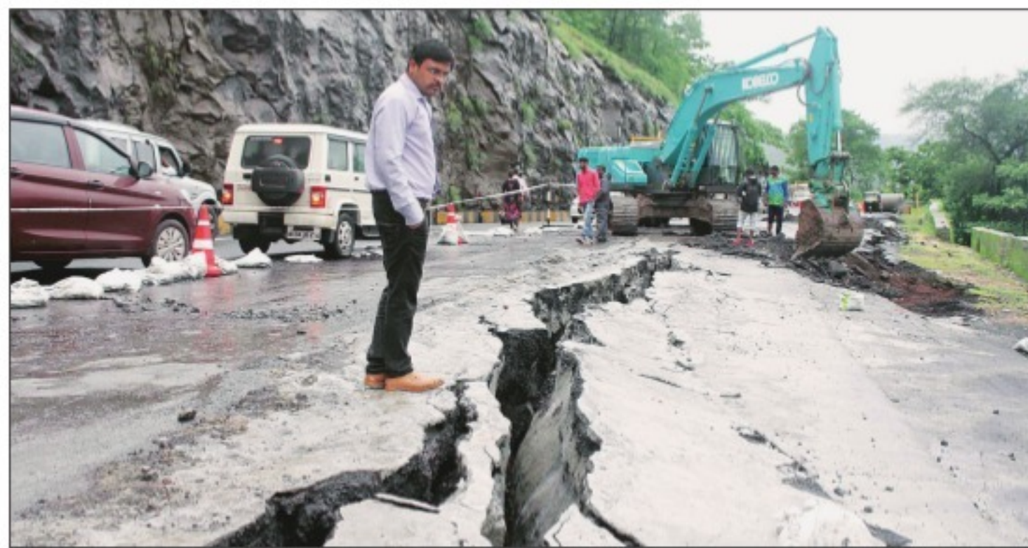
The Mumbai-Nashik highway in Maharashtra's Kasara Ghat was reduced to a single-lane road after developing major cracks due to heavy rainfall. Meanwhile, heavy rain and flooding wreaked havoc in Sangli and Kolhapur districts, leading to the evacuation of around 56,000 people from affected areas, and the closure of the Mumbai-Bangalore highway between Sangli and Kolhapur. Deepak Joshi
