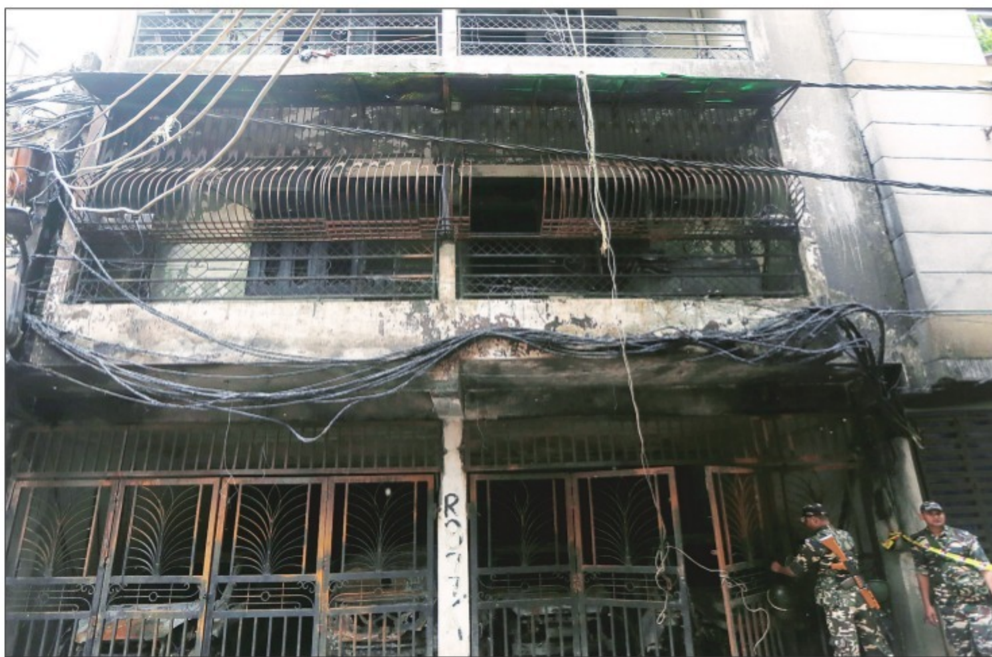
The fire broke out at the electricity meter in the parking lot of the Zakir Nagar building. Photos: Prem Nath Pandey
