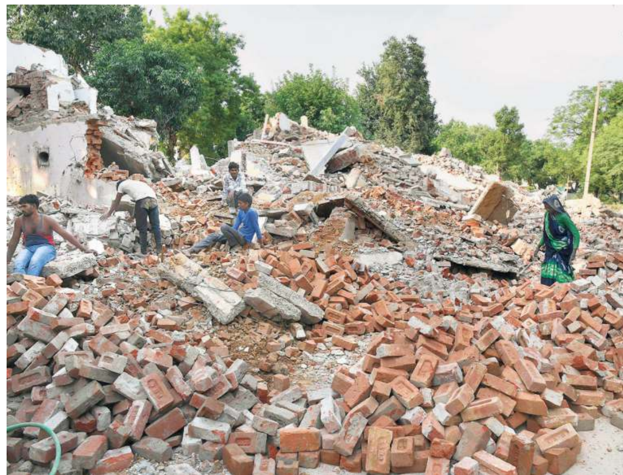
Workers at a site where a demolition drive is being carried out for a redevelopment project at Netaji Nagar Block-F in New Delhi. • SHIV KUMAR PUSHPAKAR
