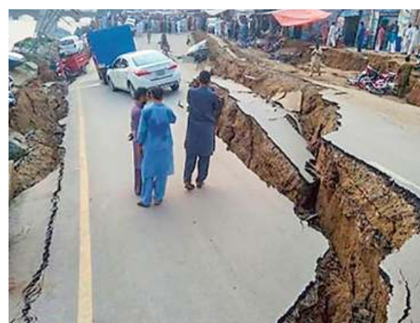
A road in Pakistan-occupied Kashmir that was damaged in the earthquake. • PTI
