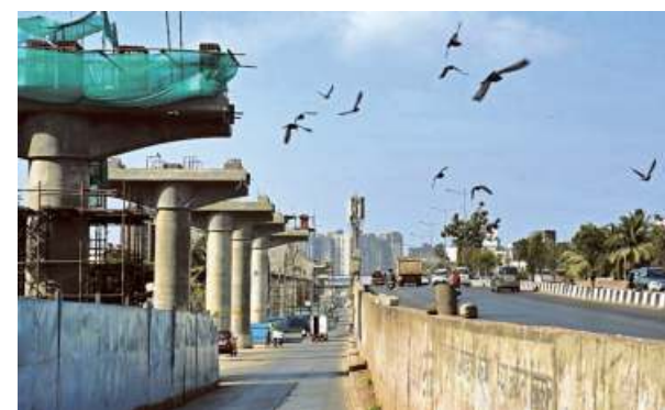
To achieve $5 trillion in GDP by FY25, India needs to spend $1.4 trillion on infrastructure. ■ ARUNANGSU ROY CHOWDHURY
