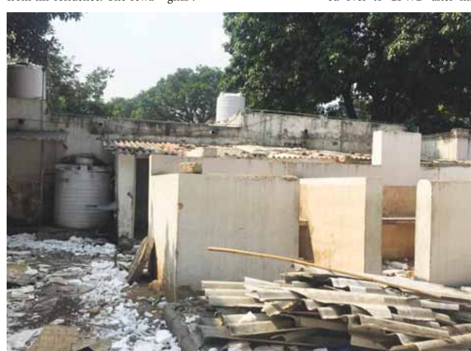
A view of partly-demolished section of the residence of former MP Rajesh Ranjan, alias Pappu Yadav, at 11A, BR Mehta Lane, in New Delhi on Thursday. Pioneer photo
