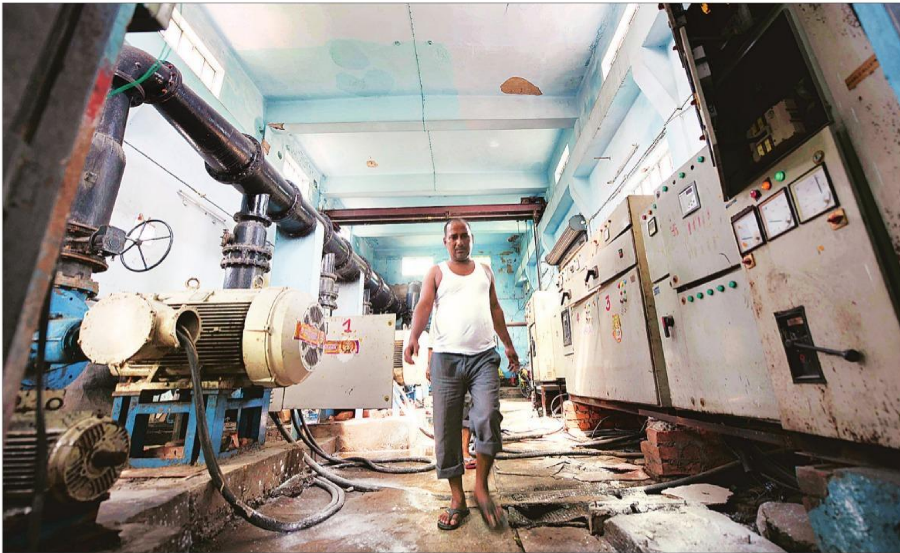
One of the four operators on the 6 am to 2 pm shift, Sharma has to ensure that the pump sets discharge water into a drainage tank, from where it is pumped out to the Rampur canal. Alok Jain
