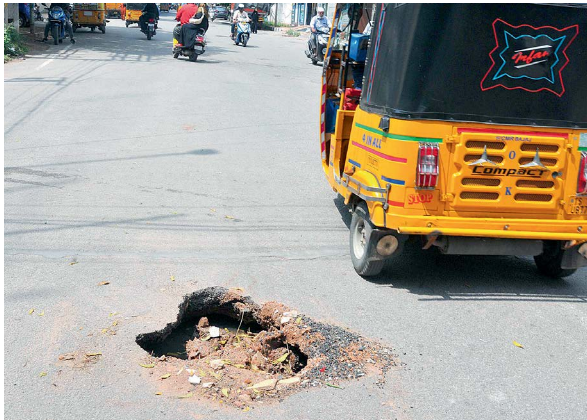
While motorists are already careful about potholes in the road, they will now need to be careful about cave in as the recent heavy rains saw quite a few roads cave in. Even the road at Akbarbagh in Malakpet too had a cave in
