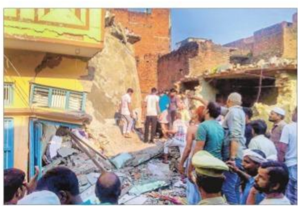
Rescue operation under way at the site of building collapse following a blast in Mau district of Uttar Pradesh on Monday. PTI
