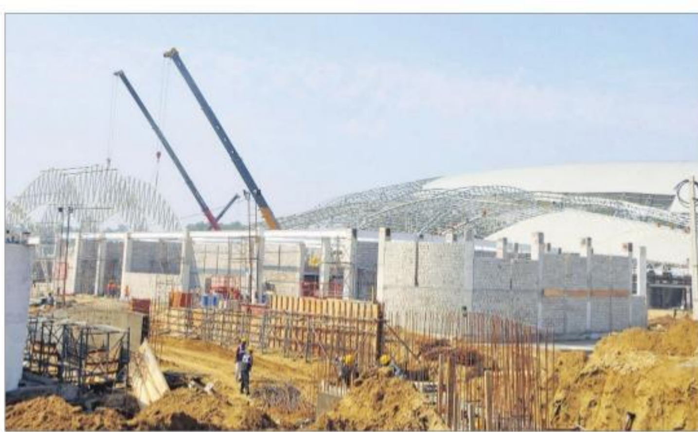
The under-construction Integrated Check Post (ICP) at Dera Baba Nanak. TRIBUNE PHOTO
