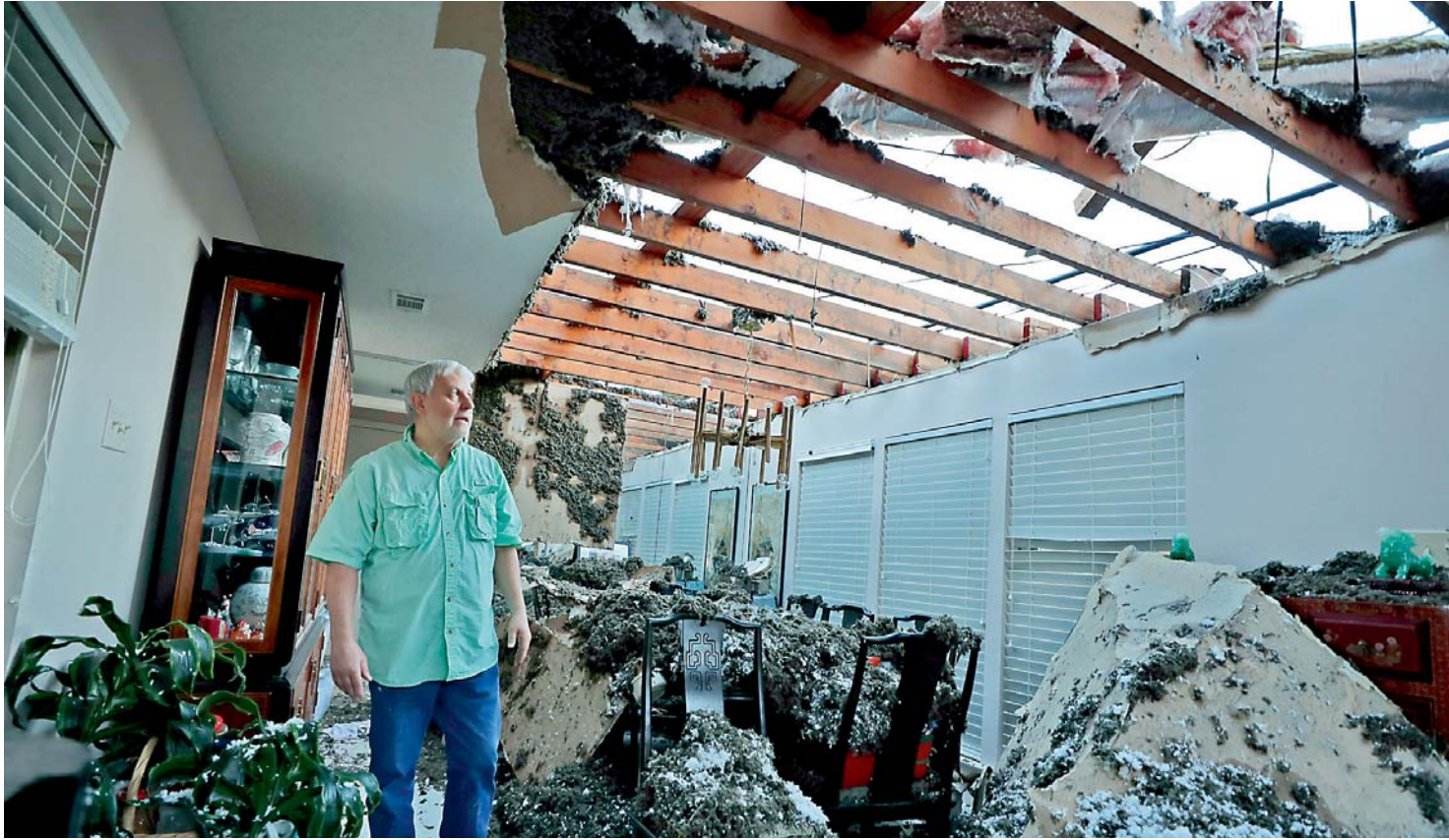
A man looks at his missing roof after his home was hit by a tornado in Richardson, Texas on Monday. A tornado tore homes and businesses apart in a densely populated areas of Dallas, where only minor injuries were reported, but a person was killed by a falling tree in northwest Arkansas as a series of storms caused chaos in several US states.
