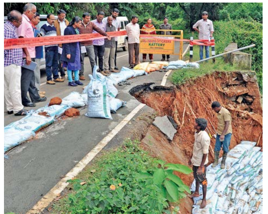
Nilgiris Collector J. Innocent Divya inspects the flood affected Ooty-Kundah road near Merland sector on Tuesday. — DC
