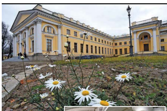
Restoration works ongoing at the Alexander Palace at Tsarskoye Selo palace museum in Pushkin outside Saint Petersburg, Russia. — AFP
