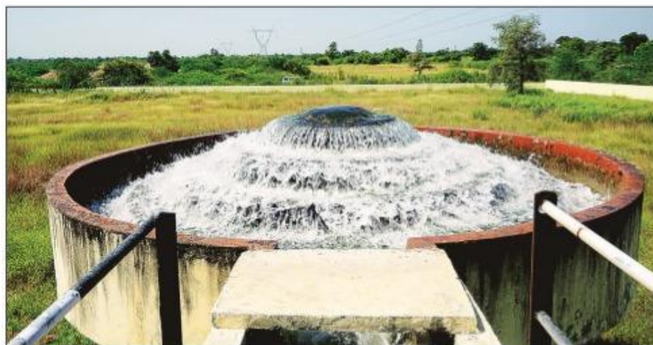
A water filtration plant of Waghodia taluka of Vadodara district Bhupendra Rana
